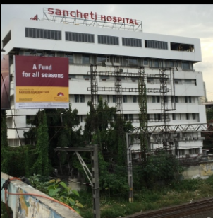
Project : Sancheti Hospital, Pune Type of Work : Hospital Building - Extension two floors (composite steel building with Civil, Interior) Quantum of Work : 25,000 Sft.
