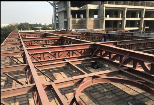
Project : Nirma University, Ahmedabad Type of Work : Canopy Quantum of Work : 155 M.T.
