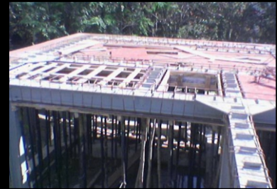
Project : United Phosphorus Ltd., Director Bungalow Type of Work : Composite Steel Structure Quantum of Work : 100 M.T.
