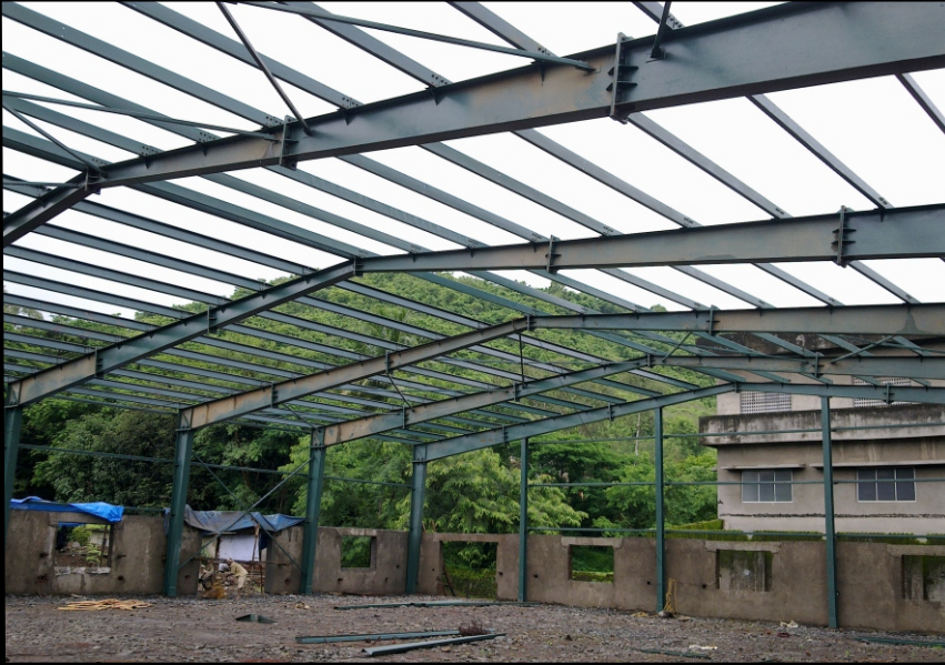
Project : Attur Enterprises Pvt. Ltd., Rasayani Type of Work : Factory Building Roof Structure Quantum of Work : 12,000 Sft.
